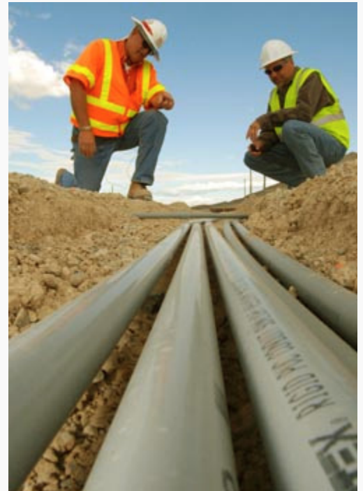
Roger Miller (Left), construction representative for the U.S. Army Corps of Engineers Los Angeles District at the Creech Air Force Base, Nev., Project Office, and Troy Fish, superintendent of Cobblestone Construction Company, inspect underground power lines March 2, 2010 where the new wing headquarters is being constructed. (USACE Photo by Lee Roberts)
