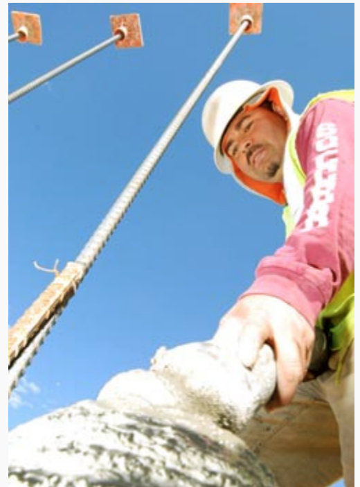
A contractor places concrete to strengthen the walls of the new dining hall. (USACE Photo by Lee Roberts)
