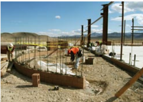
A U.S. Army Corps of Engineers contracted construction crew builds the new dining facility at Creech Air Force Base, Nev., March 2, 2010. (USACE Photo by Lee Roberts)
